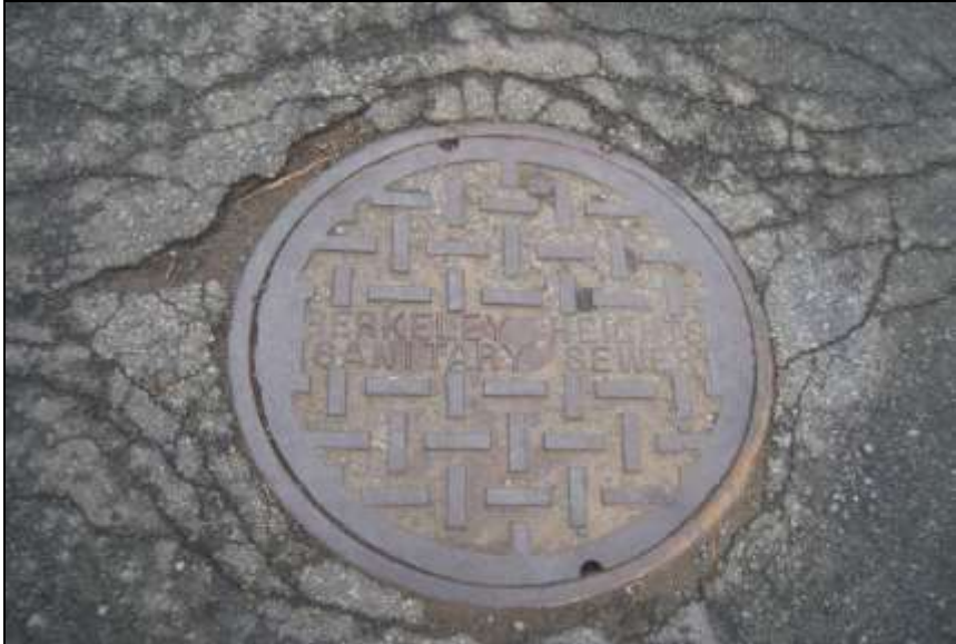
Photo # 8- Manhole cover indicating "Berkeley Heights Sanitary Sewer" just beyond the storm drain.
