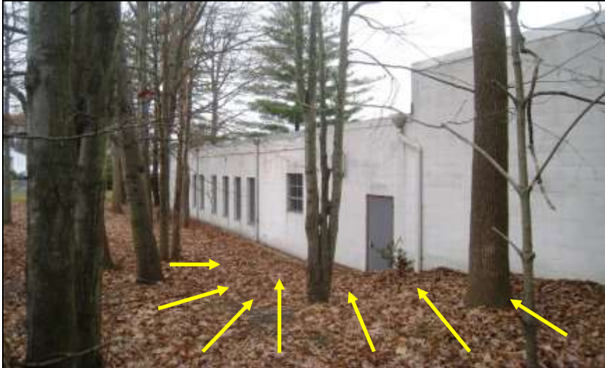
Photo # 14- SE corner of building looking toward Russo Place on right side of building. Grading knee deep in leaves and grading pitched toward rear door by print shop/mail room.
