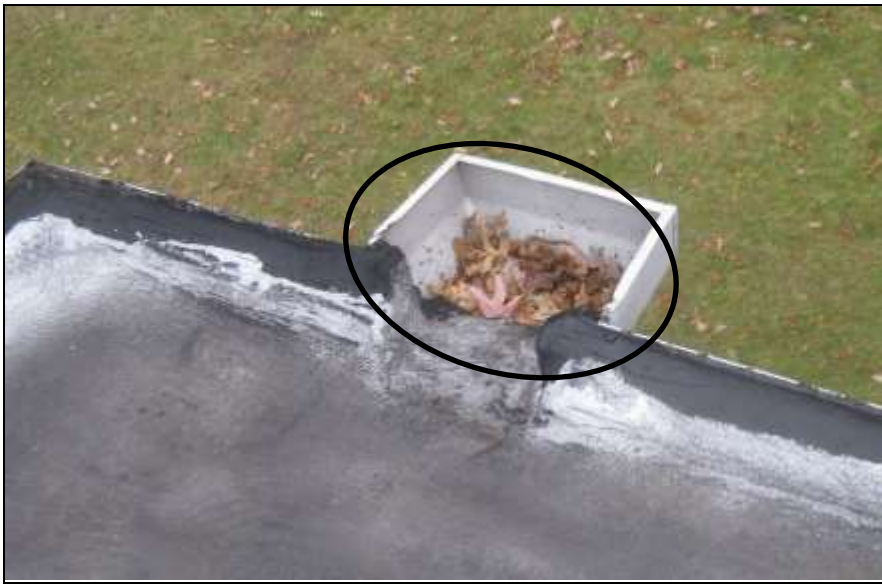
Photo # 22- Clogged scupper
