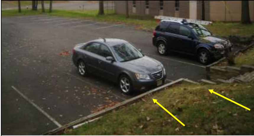
Photo # 2- Grading and water runoff onto north parking lot and rail road tie retaining walls. RR ties were leaning, failed, and infested with insect damage. There was no railing or lighting on steps; safety concern.
