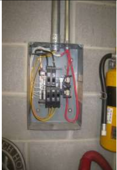
Photo # 38- Main electrical meter and 1 and 3 phase 200 amp disconnects for building.
