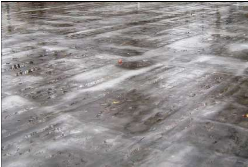
Photo # 25- Water ponding on roof.
