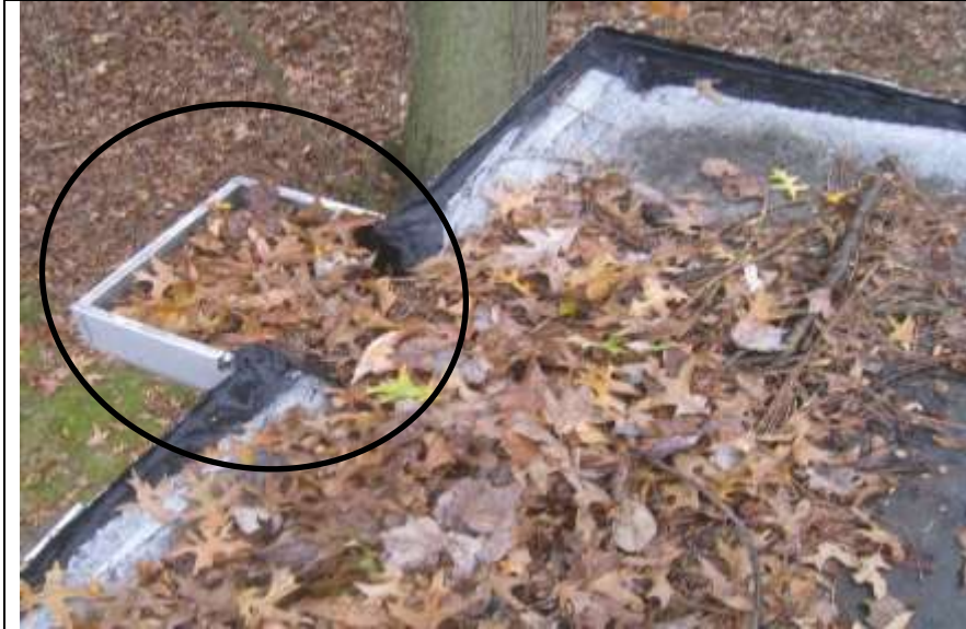
Photo # 23 – All scuppers were clogged with leaves and tree debris.
