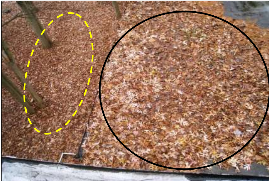
Photo # 19-. Deep piles of leaves along south wall or right side. Deep piles of leaves below among the dense trees.
