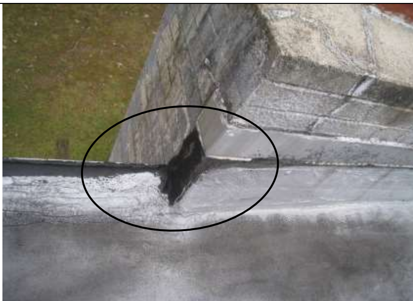
Photo # 30- Example of tarred flashings; vulnerable areas for leaks.
