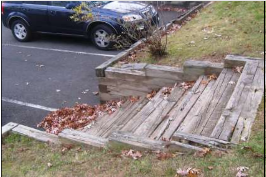
Photo # 4 – Rotted RR tie steps; no railings and lighting over steps. No railings along RR tie retaining walls.
