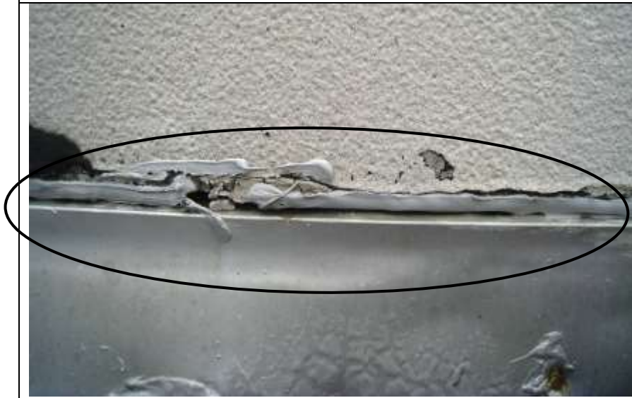
Photo # 29- Typical of split or open seams on metal flashing; water entry points.
