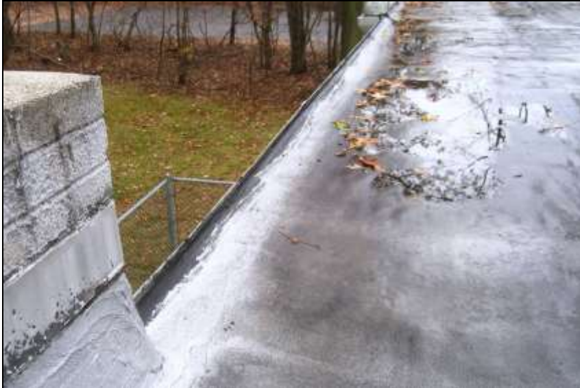
Photo # 26- Water ponding on roof.
