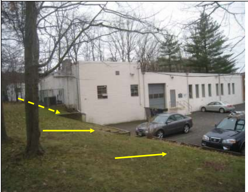
Photo # 3- Water drainage from east end property contributing to failed and rotted rail road ties.
