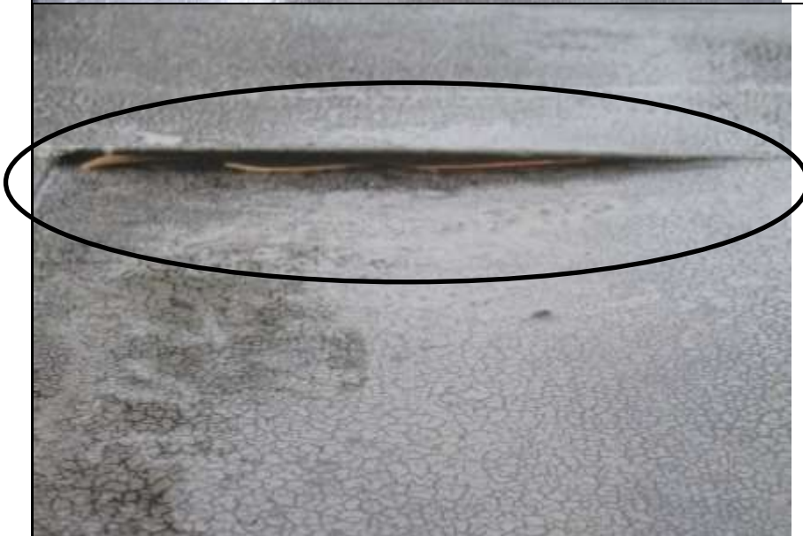
Photo # 27- Typical example of lifted seams; water entry points.
