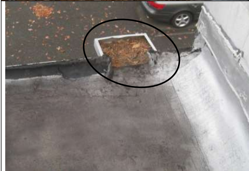
Photo # 21- Clogged scupper and cracks on tarred flashings.
