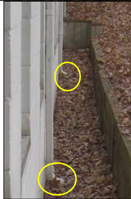
Photo # 15- South side depicting RR tie retaining wall leaning and WDI damage.
