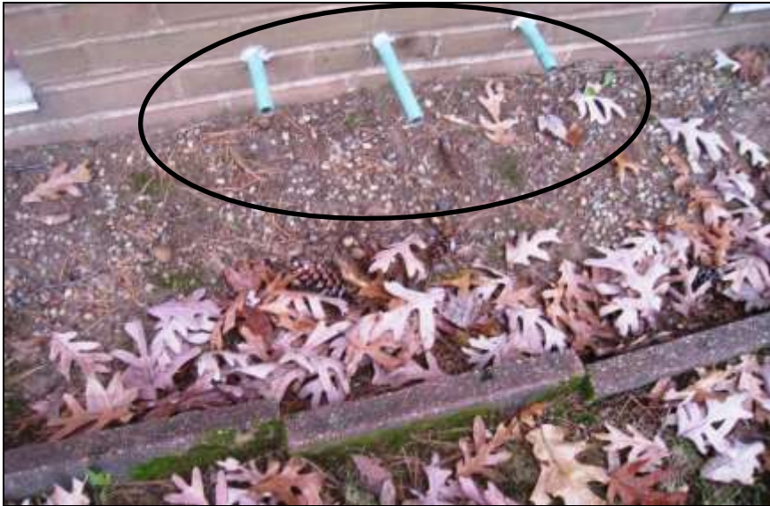
Photo #13- Same area as #12 above depicting 3 condensate tubes from the Valance cooling system.
