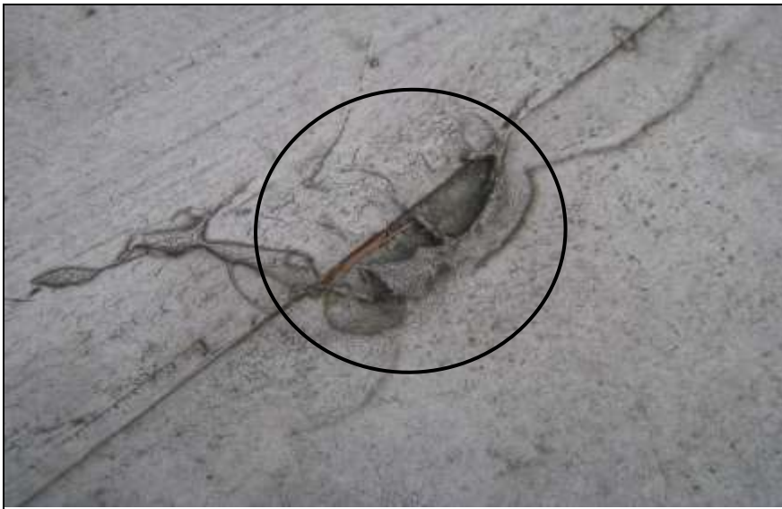
Photo #28- Typical example of puncture, digs or holes; water entry points.
