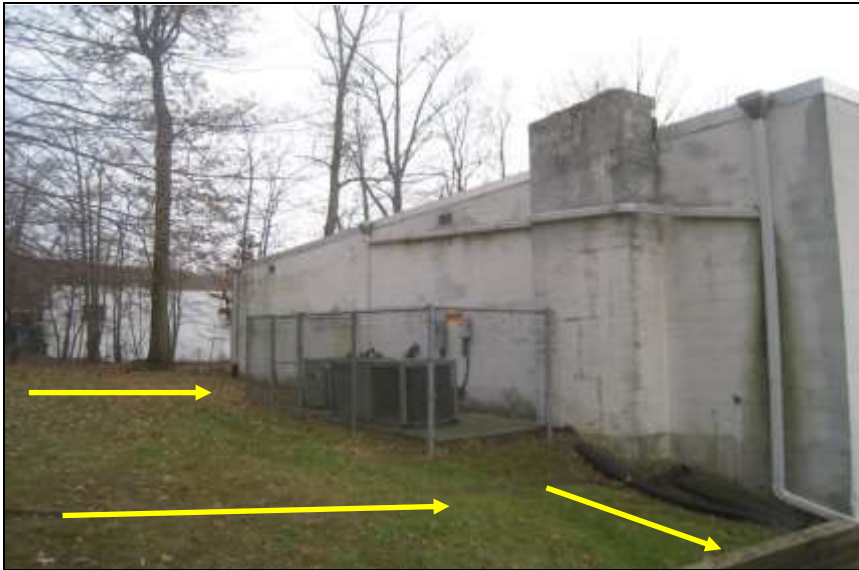
Photo # 1- (Topology) General slope downward from rear or east property toward Russo Place. Water draining toward rear of building, and parking lot on north side and around south corner of building. Arrows indicate general flow or drainage.
