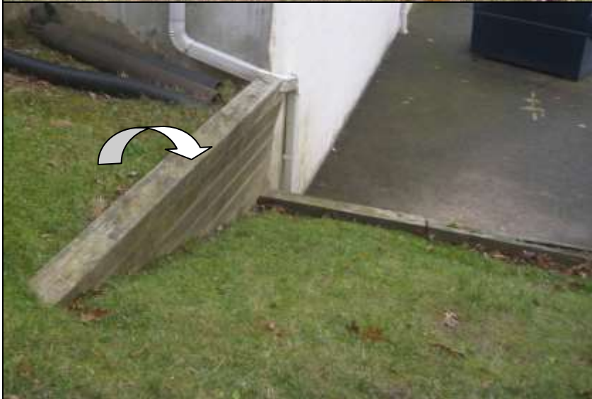
Photo # 5- RR tie retaining wall leaning or failed. Wood ties on property were rotted and had insect and water damage.
