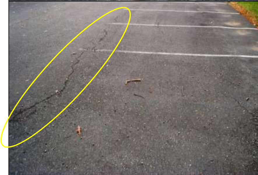
Photo # 9- Parking lot has settling or drying cracks and faded parking space markings.
